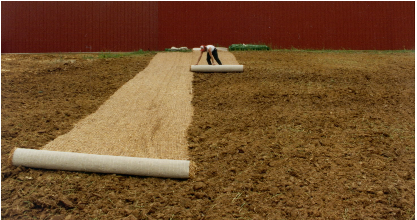
Step Five—Starting at the crest of the slope, roll the RECP down the slope in a controlled manner.
