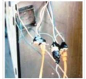
These cords are improperly wired directly to the electrical circuit, are not protected by a GFCI, and are two-wire cords that are not grounded and not rated for hard- or extra-hard service.
