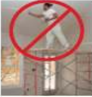
This worker is at risk because there is no fall protection.
