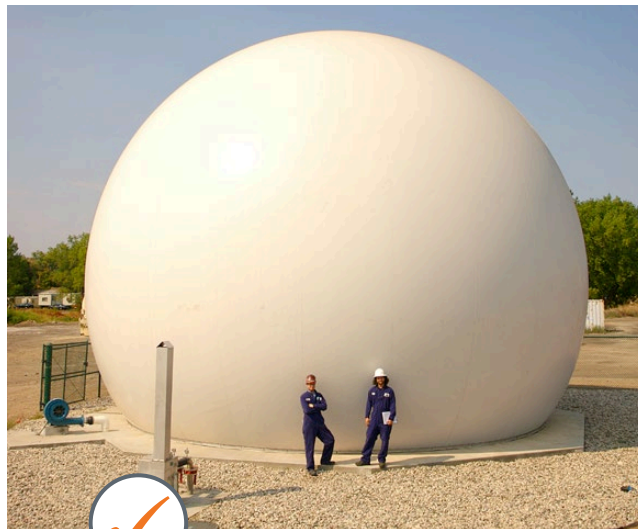
Biogas from process water treatment is captured in methane balloons before being piped to the CHP system. Photo courtesy of New Belgium Brewing Company
