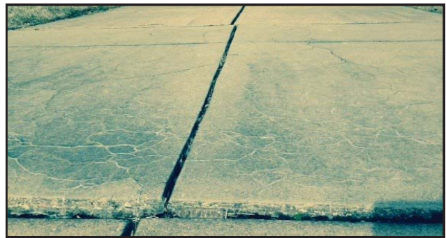
ASR Cracking and Expansion in Sidewalk
