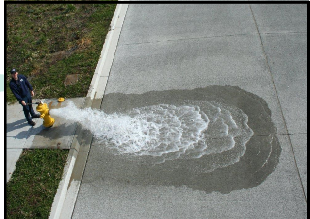
Pervious Concrete Infiltrates Water
