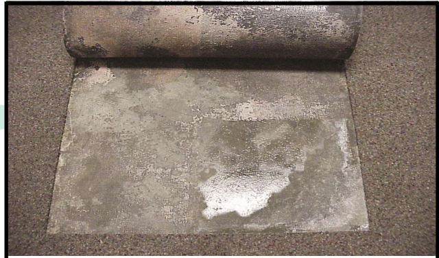
Moisture-related Floor Covering Failure (PCA image)
