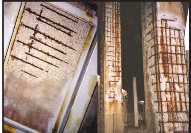
Reinforcement Corrosion in Structures
