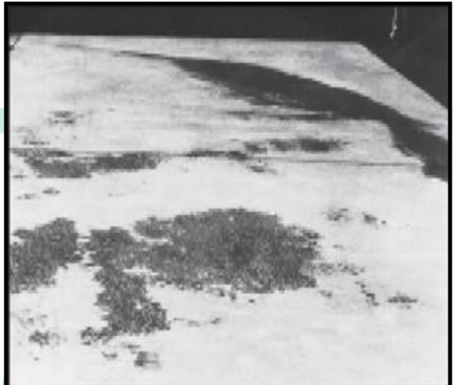
Discoloration on a Slab on Ground
