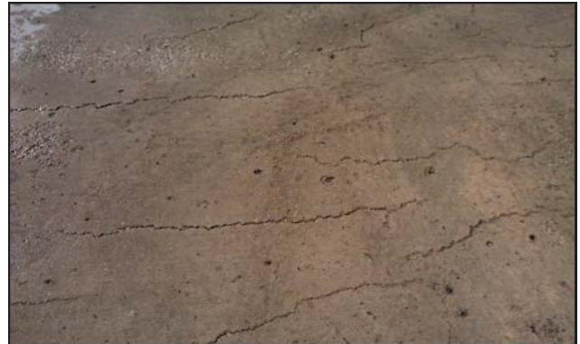
Plastic Shrinkage Cracks
