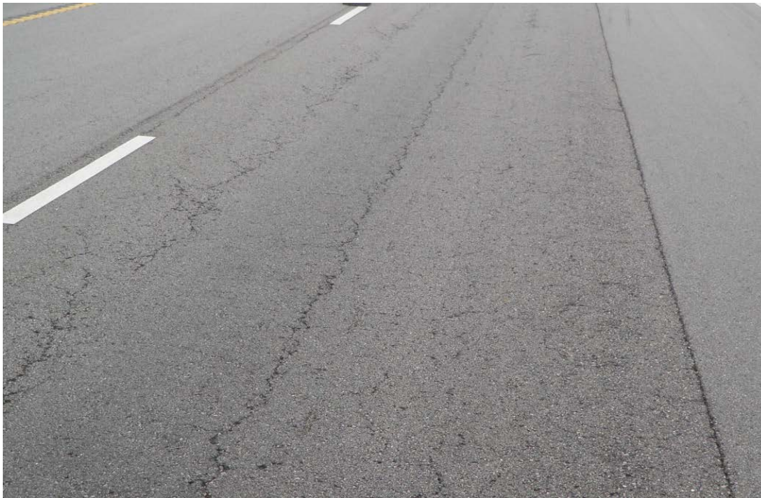
Figure 2. Fatigue cracking on a Missouri pavement.
