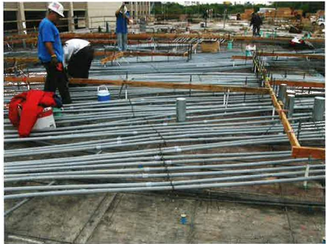
Fig. 8.4—Large group of conduits in slab.
