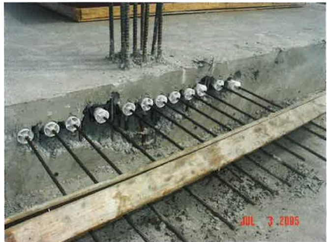
Fig. 8.5—Poor concrete consolidation in anchorage area.
