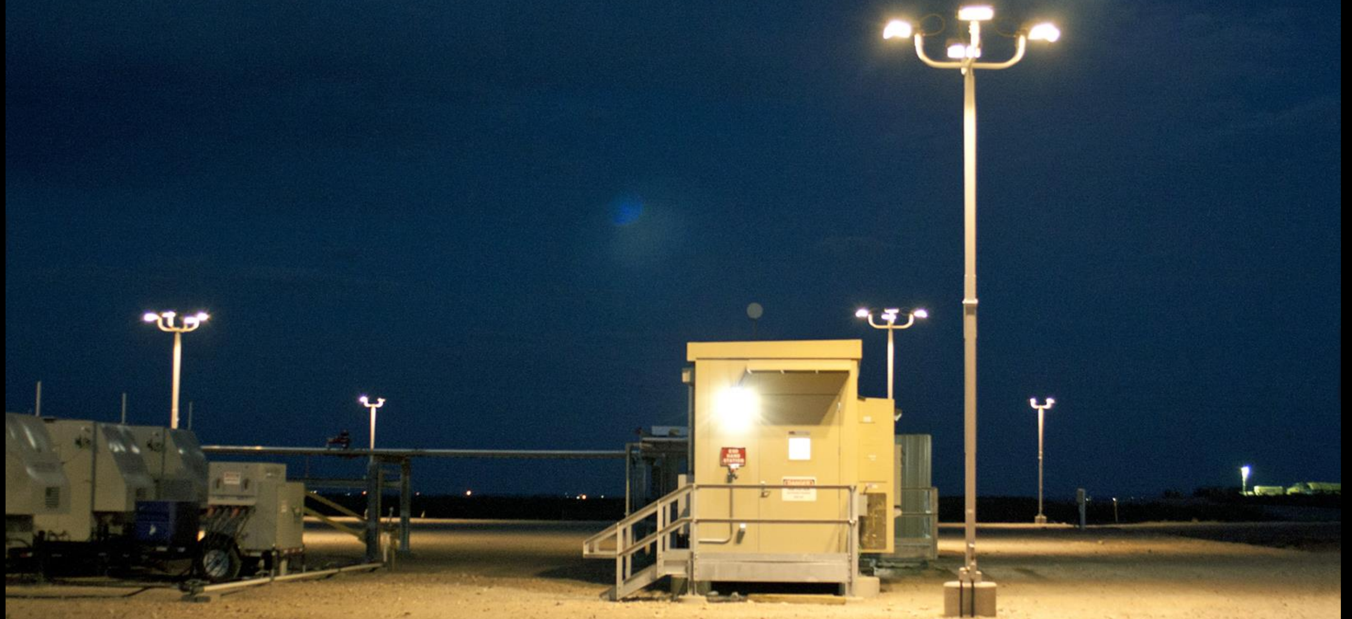
Apache Corporation Compressor Station
