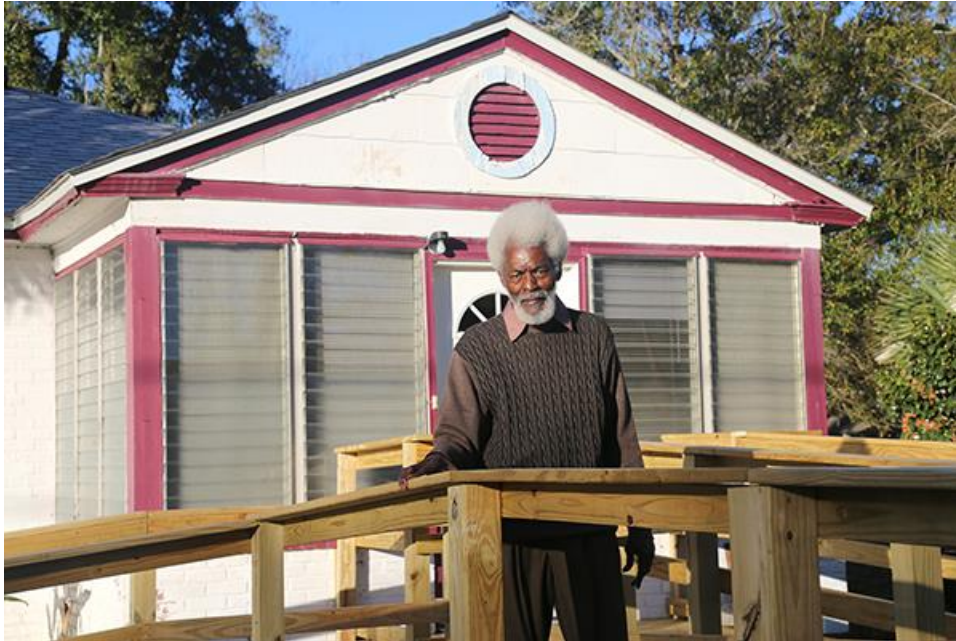
Before and after photos of the wheelchair ramp at Hoza and JoAnn Turner's home
