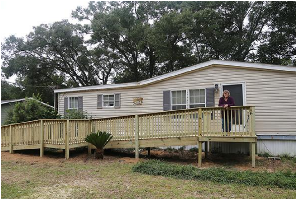
Escambia County resident Charlotte Swearingen on her new porch and wheelchair ramp installed through the Escambia County Wheelchair Ramp Program.
