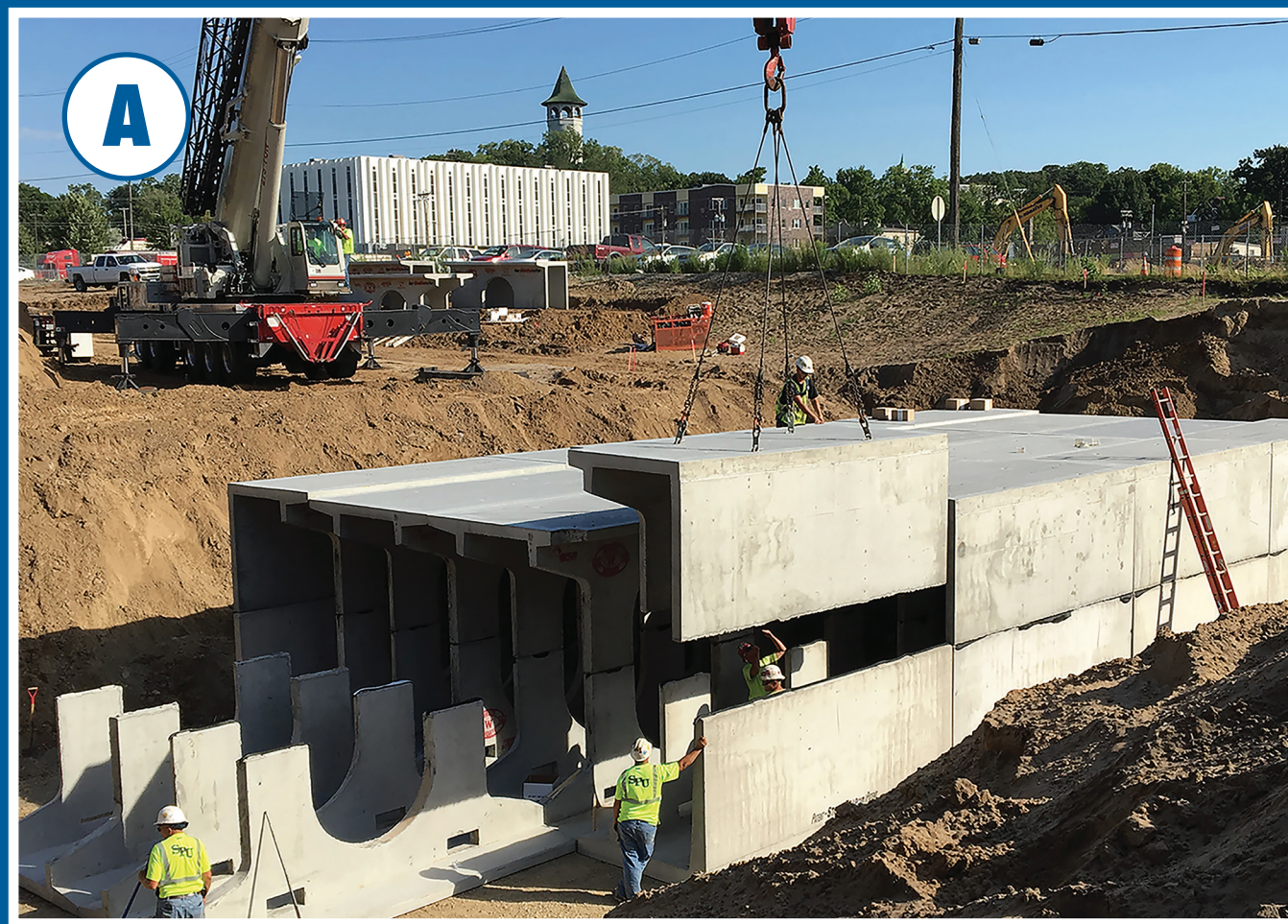
A Two large biofiltration basins collect and treat runoff that is conveyed to a 207,000-gallon underground cistern for irrigation storage and treatment.
