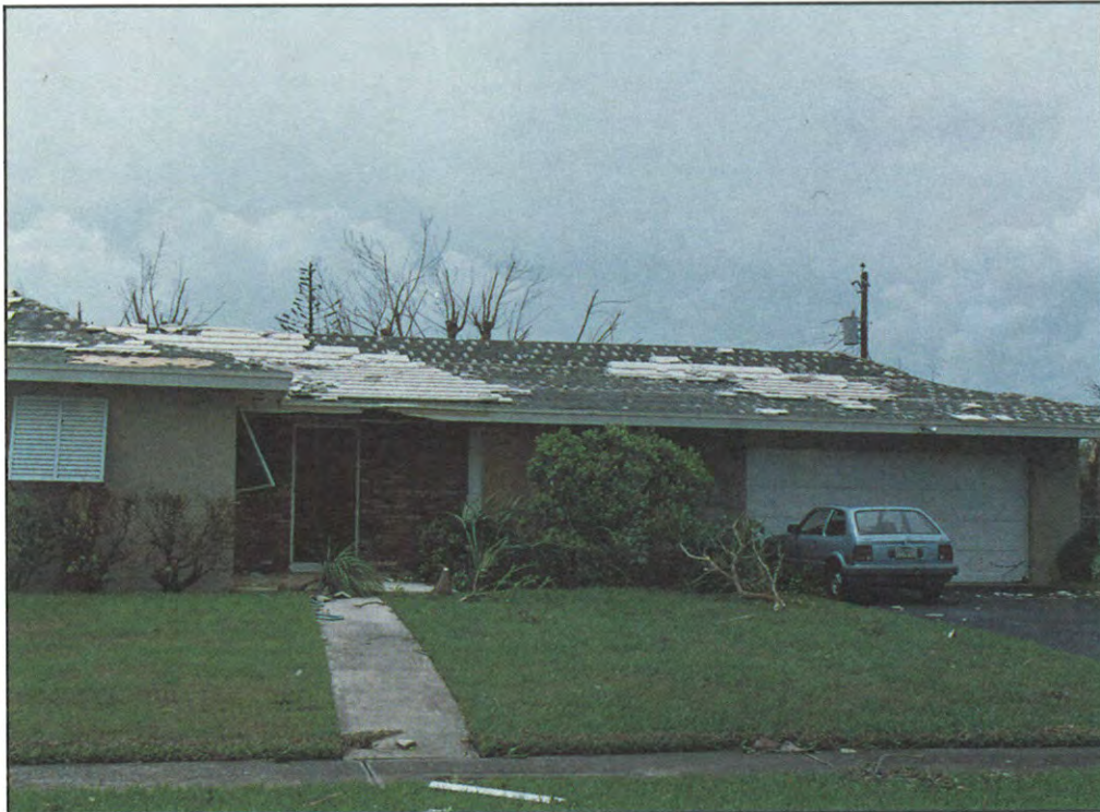
FIGURE 32. Failure of extruded concrete flat tile roofing. Bond failure between tile and mortar and between mortar and underlayment was observed.
