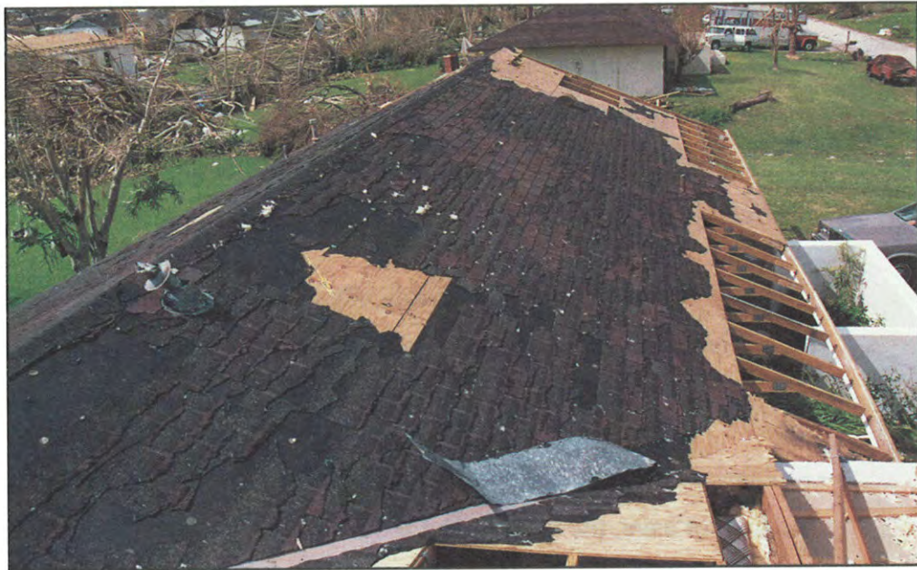
FIGURE 30. Composition shingle and underlayment failure.
