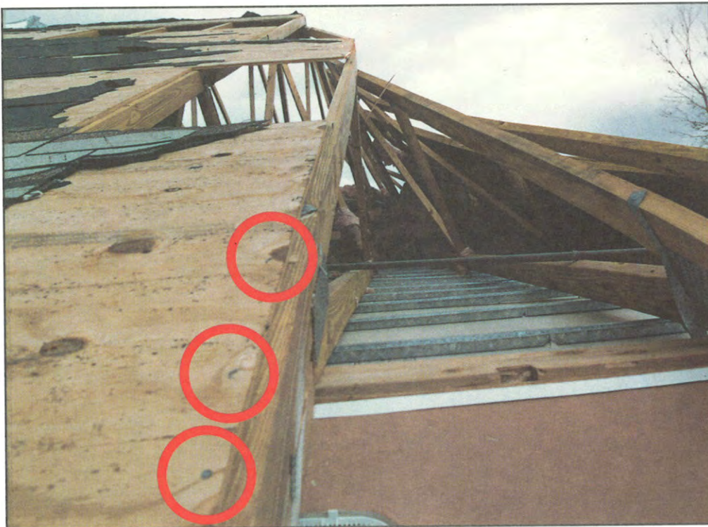
FIGURE 57. Sheathing only tack-nailed.
