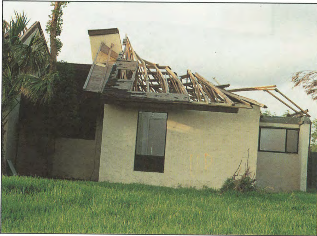
FIGURE 14. Roof structure failure due to inadequate bracing.
