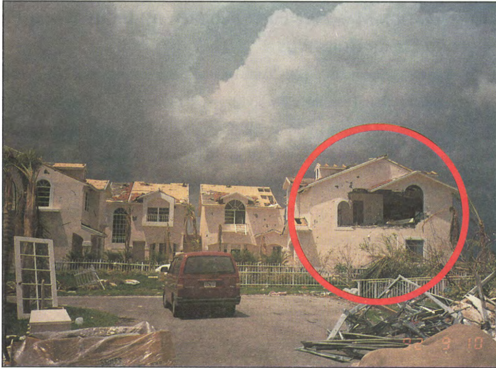
FIGURE 16. Two-story masonry buildings. Lack of continuous tie-beam led to failure of wall that was already weakened in design by window openings.
