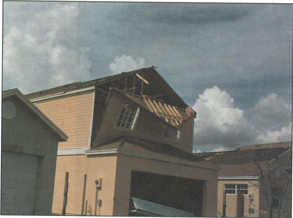
FIGURE 58. End wall failure. Example of lack of load transfer capacity after separation.
