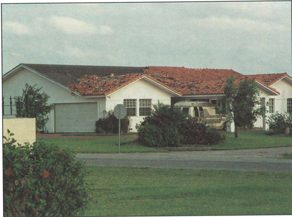
FIGURE 36. Failure of barrel tile roofing. Bond failure between underlayment and mortar and between mortar and tile was observed.
