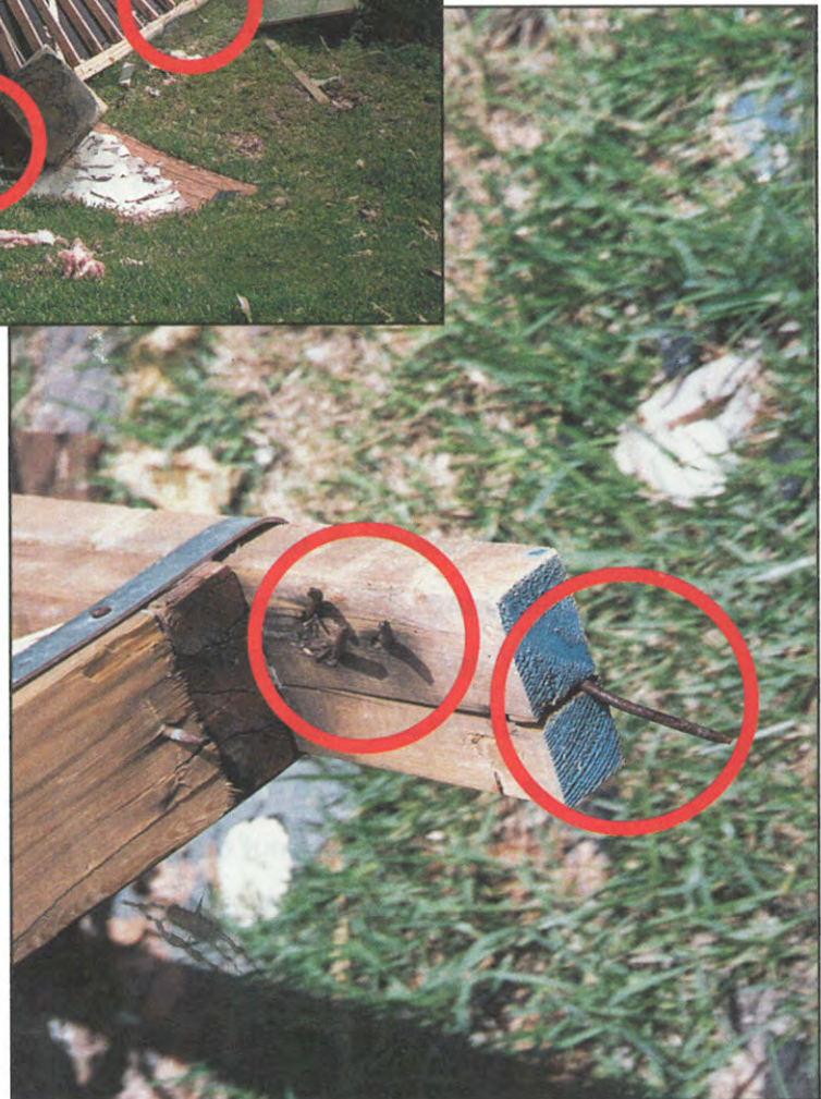
FIGURE 5. End of exterior non-loadbearing wall top plate. Transfer of forces on entire wall depended on a limited number of nails.
