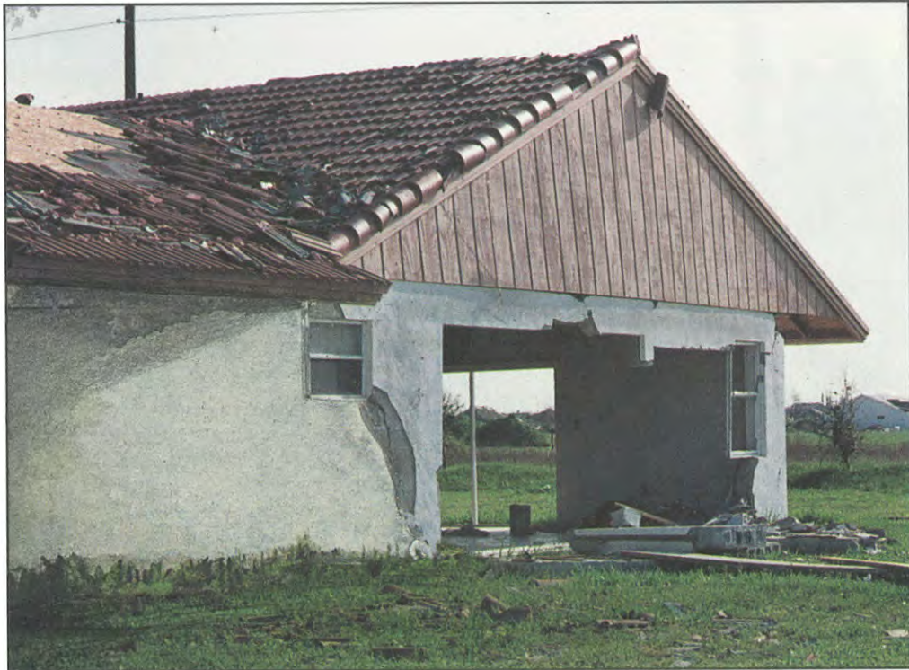
FIGURE 15. Masonry construction building. Wall separated from building envelope due to inadequate vertical wall reinforcing in connection to horizontal tie-beam.
