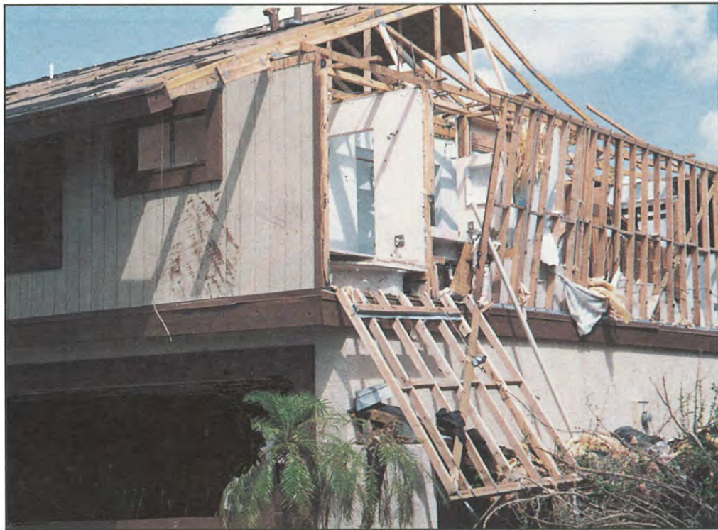
FIGURE 18. Second story wood framing (on first story masonry). End gable and wall failure.
