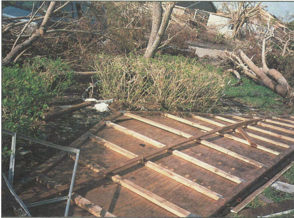
FIGURE 6. Entire wood gable separation. Bracing connection, if completed, may have prevented this from occurring.
