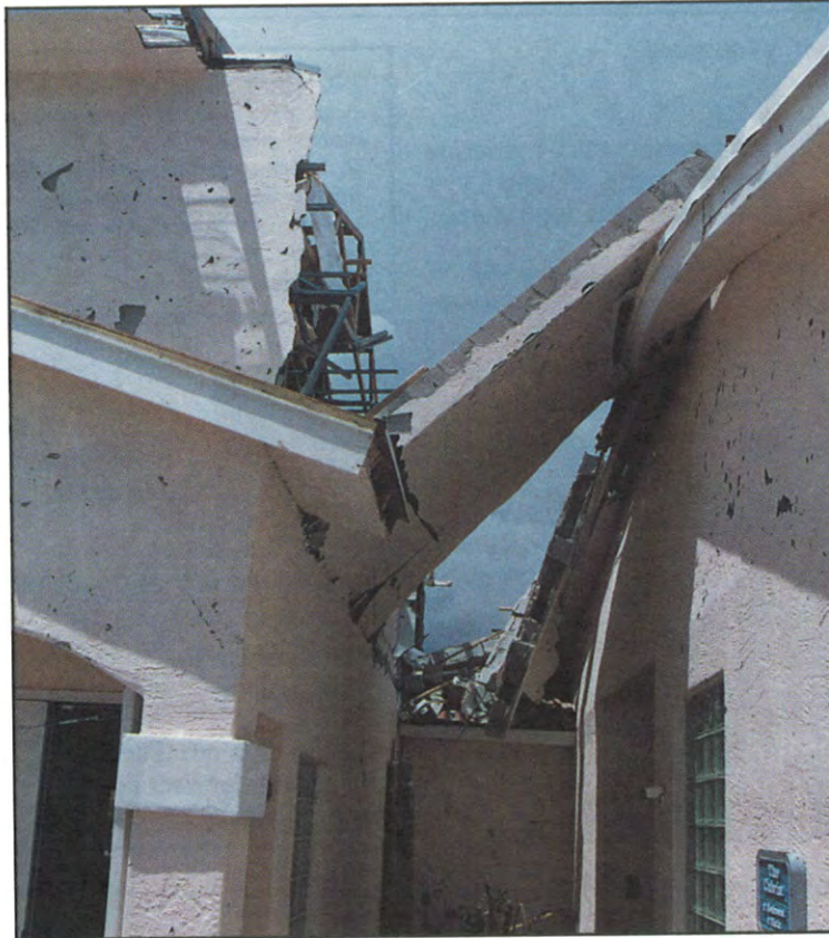
FIGURE 67. Firewall separation . Results from building corners being discontinuous with tie- beams. (See Figure 68 for side view)
