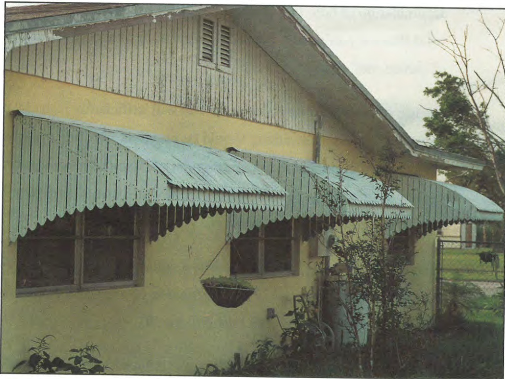
FIGURE 40. Roof gable louvered venting and convertible awning/storm shutters.
