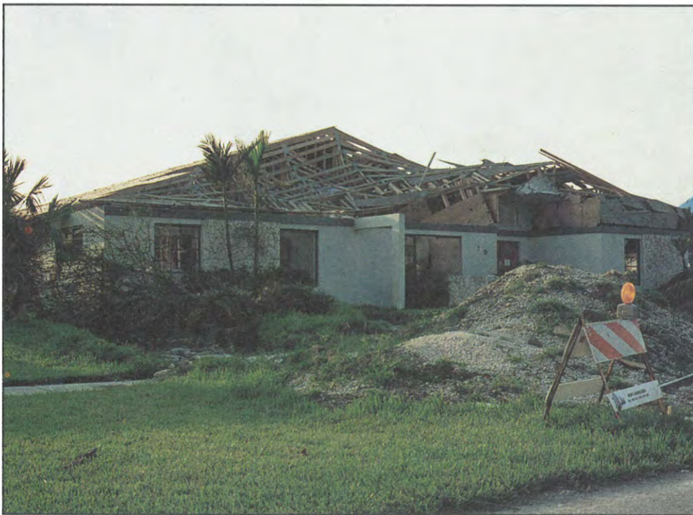
FIGURE 7. Typical gable failure. Inadequate bracing support and ridge blocking evident in inward collapse.
