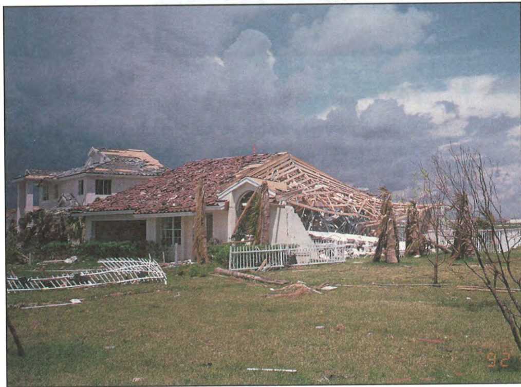
FIGURE 13. Roof structure failure due to inadequate bracing.
