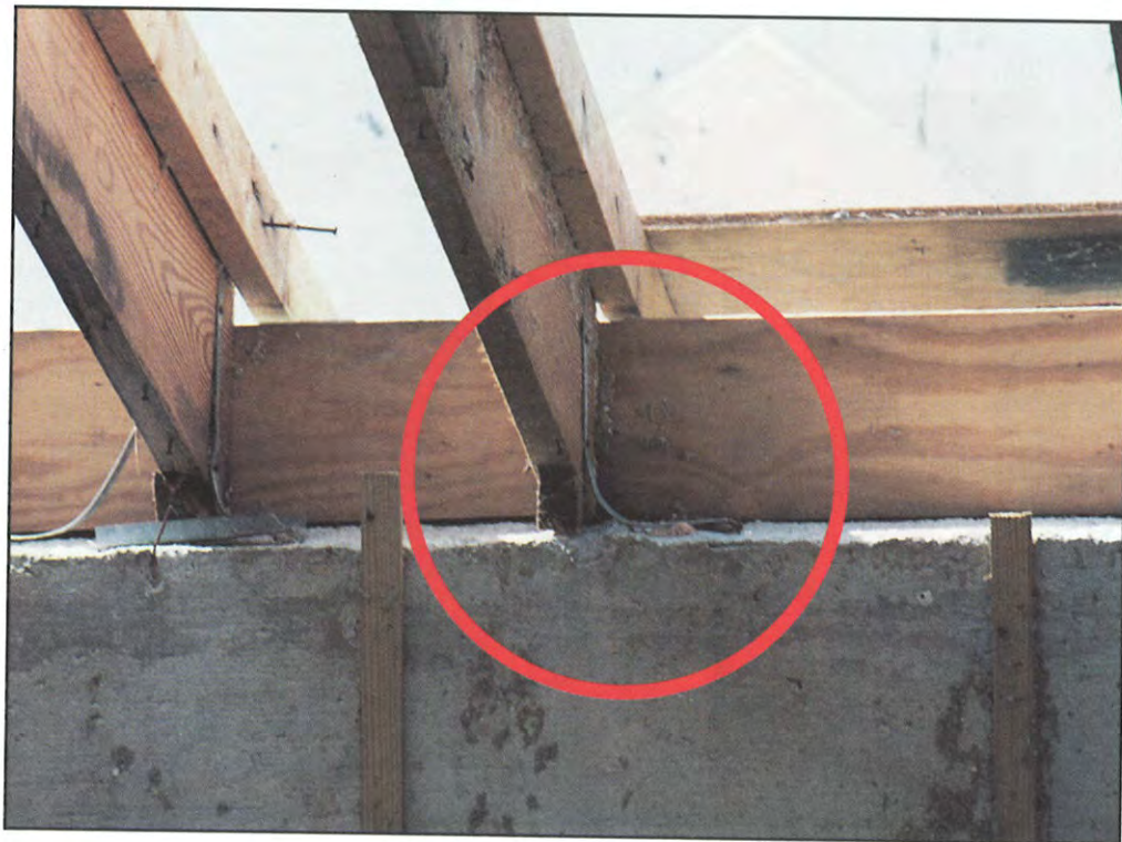
FIGURE 70. Improperly located masonry-wall-to-wood-frame straps.
