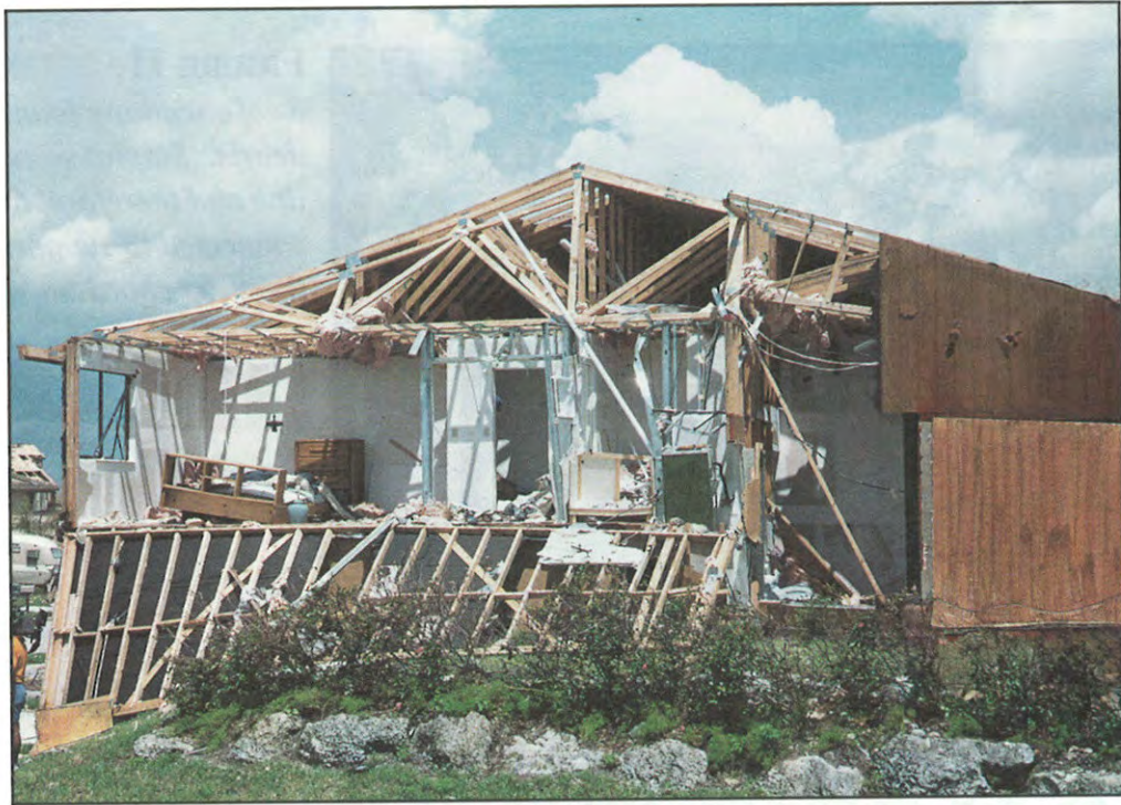
FIGURE 12. End wall failure of typical first floor masonry/second floor wood-frame building. Truss bridging and lateral bracing, and adequately installed roof sheathing, would have greatly reduced the likelihood of such a failure.
