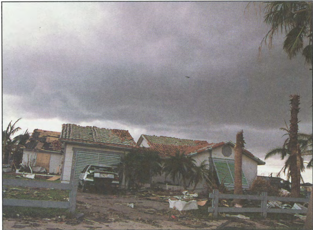
FIGURE 24. Typical roofing failure. Failure between tiles and mortar pads.
