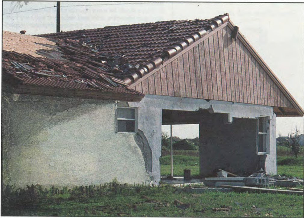
FIGURE 63. Example of masonry construction. Wall separated from building envelope due to inadequate vertical wall reinforcing in connection to horizontal tie-beam.
