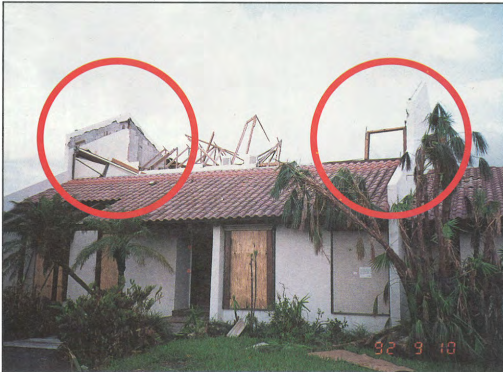
FIGURE 17. Two-story masonry building. While forces were sufficient to blow off entire roof structure, continuous masonry gables held.
