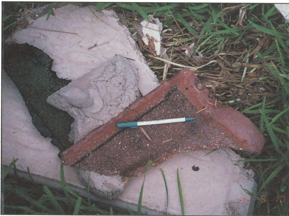
FIGURE 22. Typical failure of roof sheathing-to-underlayment attachment. (Bond between underlayment and mortar pad, and between mortar pad and tile effective.)
