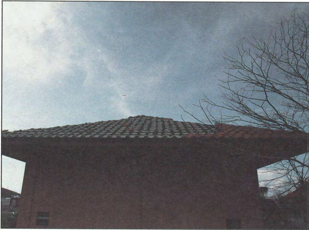
FIGURE 34. Failure of "S" tile roofing. Bond failure between mortar and tile was observed.
