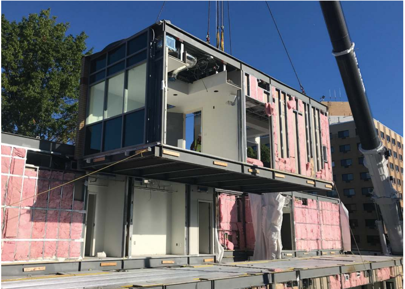
Vanderbilt Family Health Clinic installation from Axis Construction Corp. and NRB, Inc.
