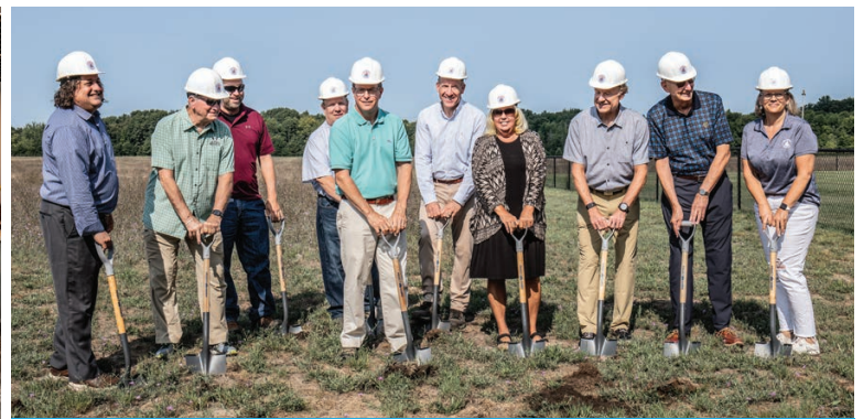
Ground breaking ceremony celebrating the construction of a pickleball complex at the Community Park in Park Township.
