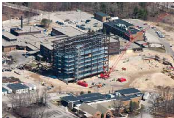
Aerial image of Mercy Health construction in Muskegon. Photo credit: Marge Beaver, Photography Plus, Muskegon, MI.
