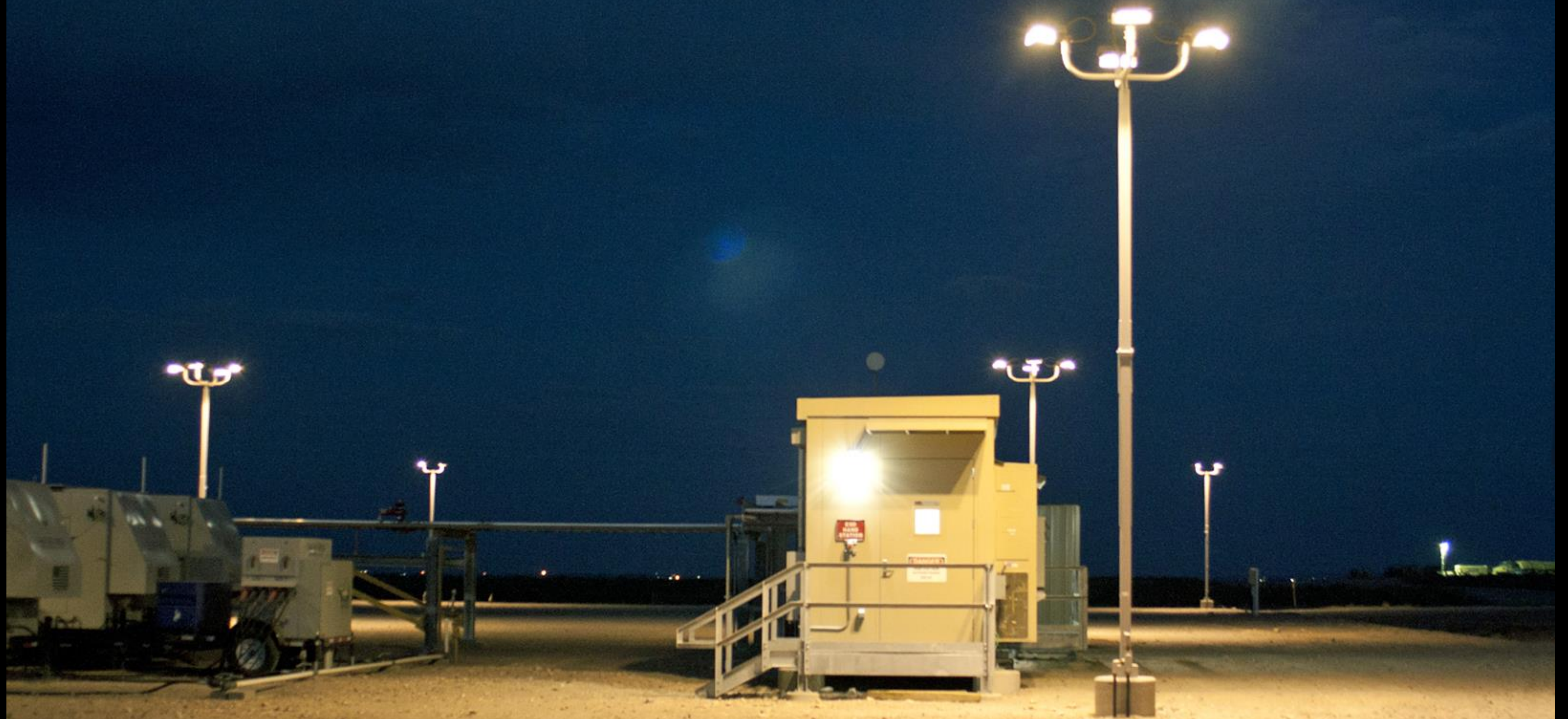
Apache Corporation Compressor Station
