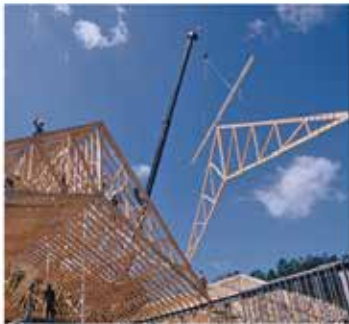
Roof & Floor Trusses
