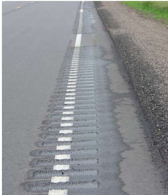
Figure 11. Rumble stripe during construction in Iowa. (Note: edge lines are repainted after rumble stripe cut.)
