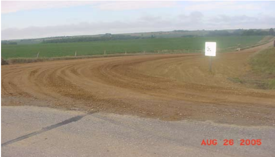
Figure 29. Alteration of vertical alignment to improve sight distance at the intersection of two county roads in Iowa.
