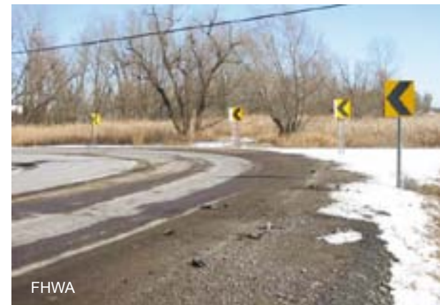
The addition of signs along local roads can lead to safety improvements at a low cost.
