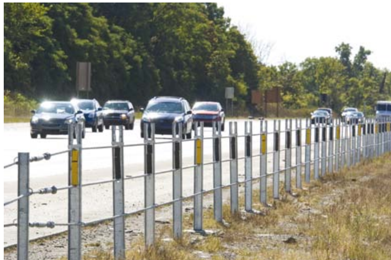
Figure 1: Cable guardrail. Photo courtesy of Michigan DOT Photography Unit.
