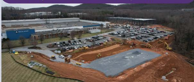
Construction underway for Delta Star's expansion - adding 149 new jobs and $30.2 Million in capital investment.
