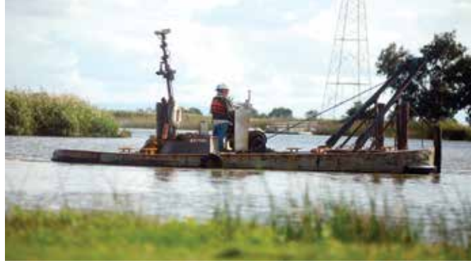
AARON ROSENBLATT/DAILY REPUBLIC Workers move their boat in position to dredge in front of the Solano Yacht Club along the Suisun City Waterfront, Sept. 18, 2019.
