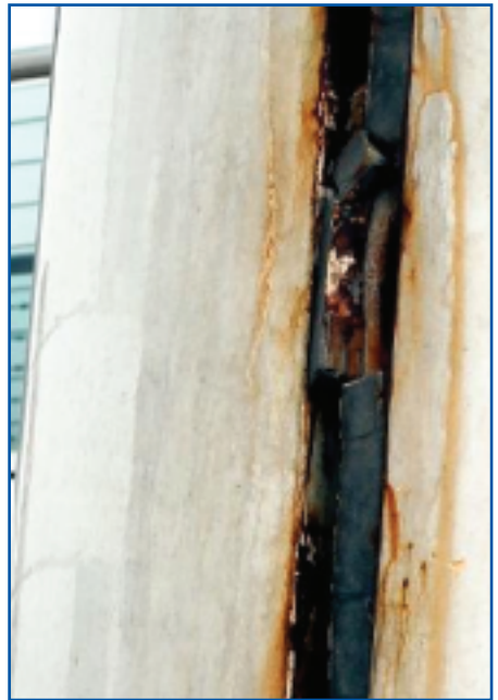
Figure 1. Corrosion to steelwork caused by water entering through a failed joint sealant.
