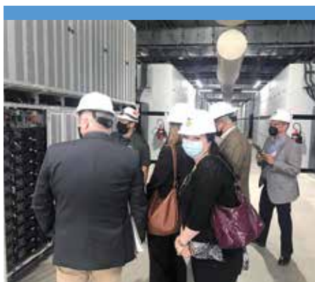
Salinas Mayor Kimbley Craig tours the Vistra facility with other local elected officials.
