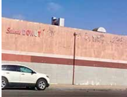
Blighted buildings in the City of Salinas.
