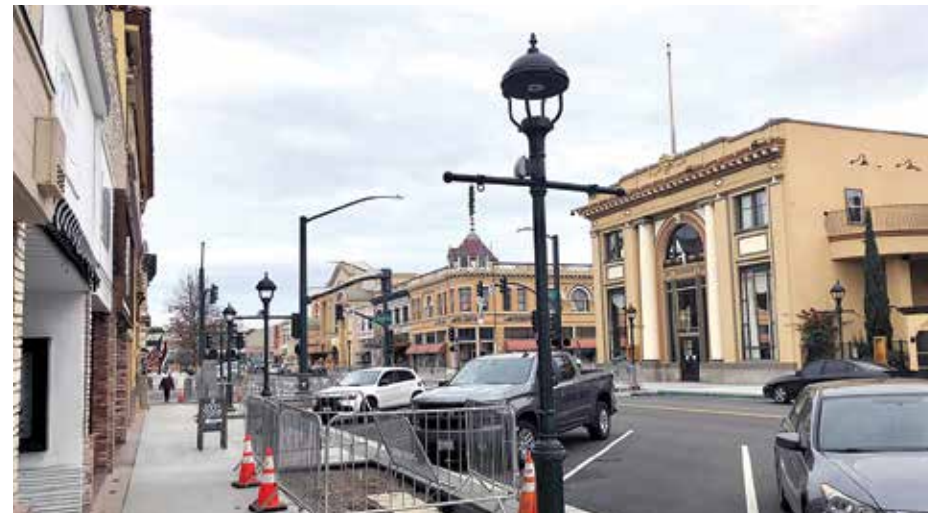
Two-way traffic is now moving on 200 block of Main Street as Main Street Streetscape Project continues
