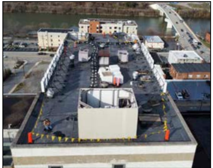
Sutter Roofing and Metal Company, Inc. of Clarksburg completed the roof renovations on the project.
