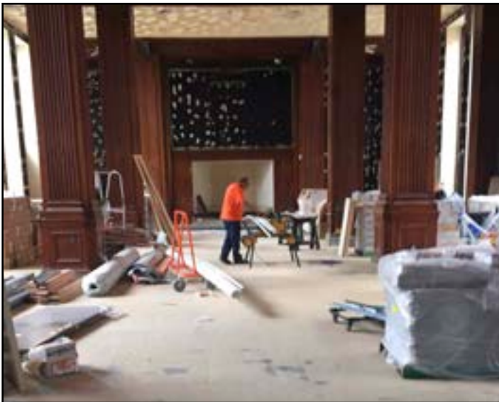
Workers from Jarrett Construction Services, Inc. work on the new ballroom at Hotel Morgan.
