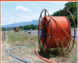
BROADBAND ACCESS $600 MILLION
